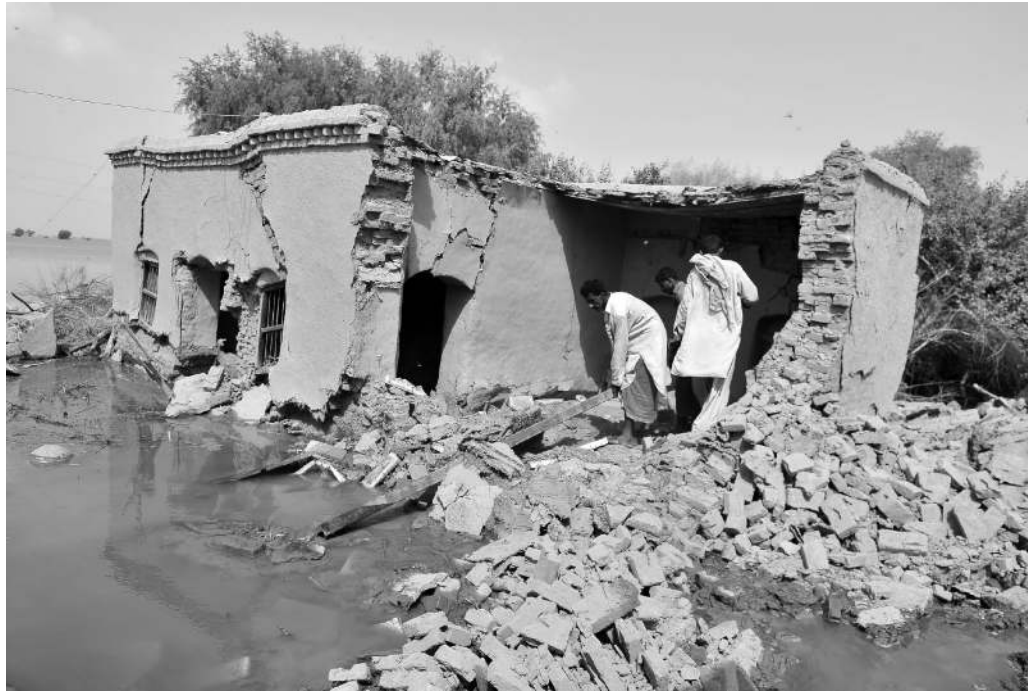
Earthquake Damage in Pakistan (2010)
